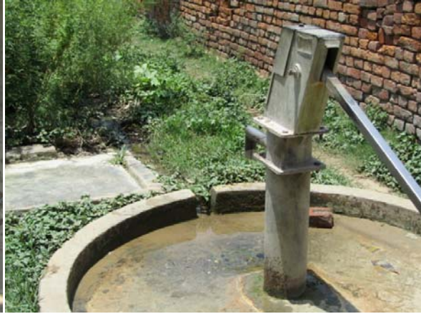
Faulty drainage is found near Hand Pump (in front of Mr Ram Naresh's house)
