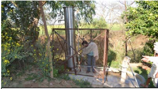
Installation of Arsenic Removal Units by Jal Nigam to provide Arsenic free water
