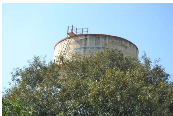
Over head tank for Ganga Pur Pipe Water Scheme
